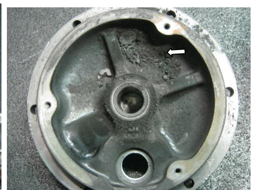
Scrape hardened brush dust from inside the CE frame, but do not scrape through the black CE frame paint coating the frame
